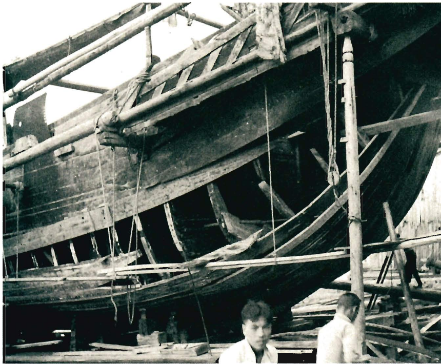
LEFT (145) A junk under repair in dry dock in Hong Kong. Four or five transverse bulkheads can be seen inside the ship and various ribs or frames are also visible. The habit of building hulls like this meant that watertight compartments were possible. If a leak occurred in one section, it could be sealed off from the rest and the ship remained afloat. Chinese ships had watertight compartments from at least the second century AD, but the idea only caught on in the West at the end of the eighteenth century. (Waters Collection, National Maritime Museum, London.)
